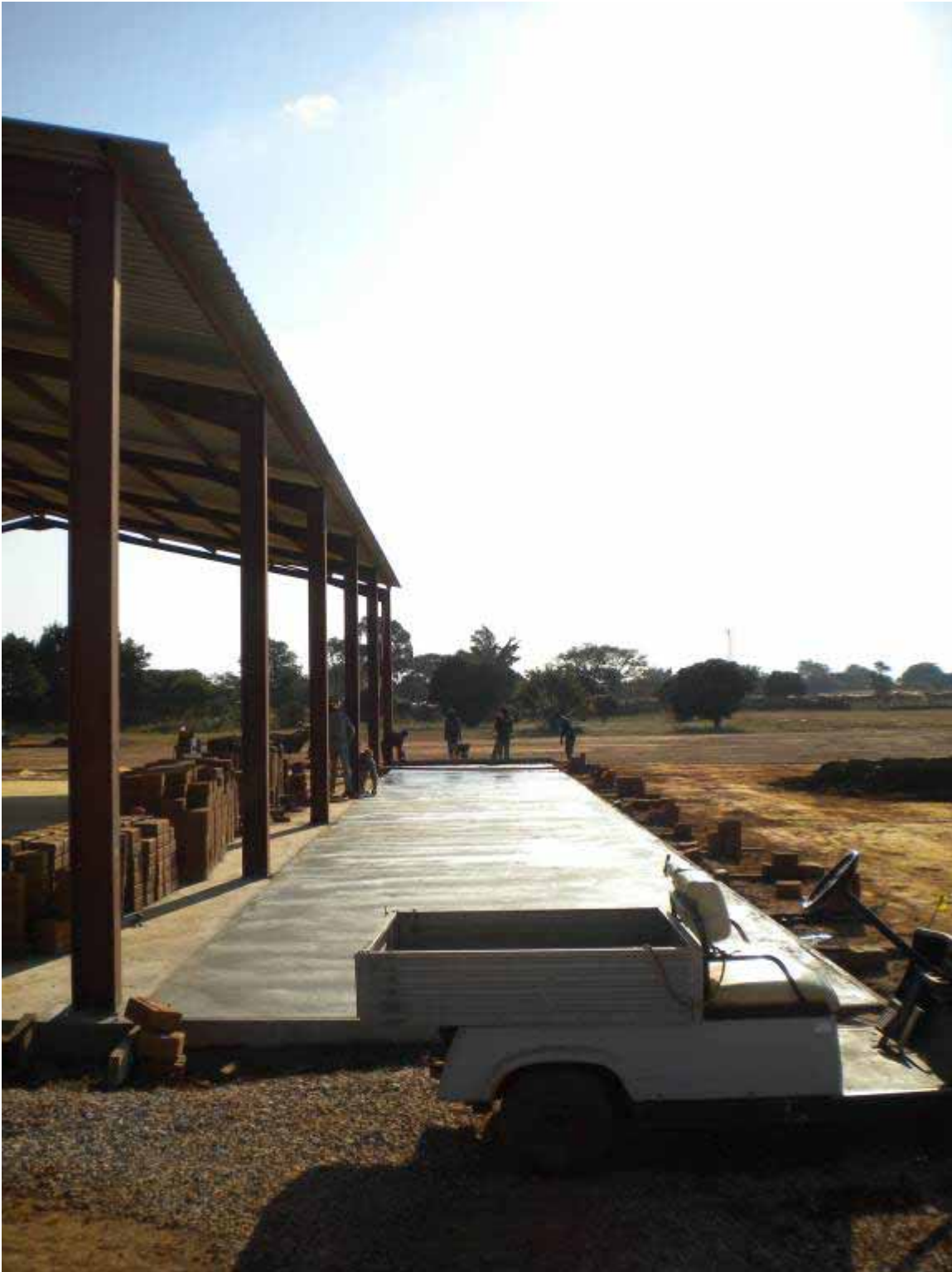
Concrete trying to dry before the sun goes down...The sun beat us.
